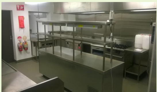
Pictured: Commercial kitchen
